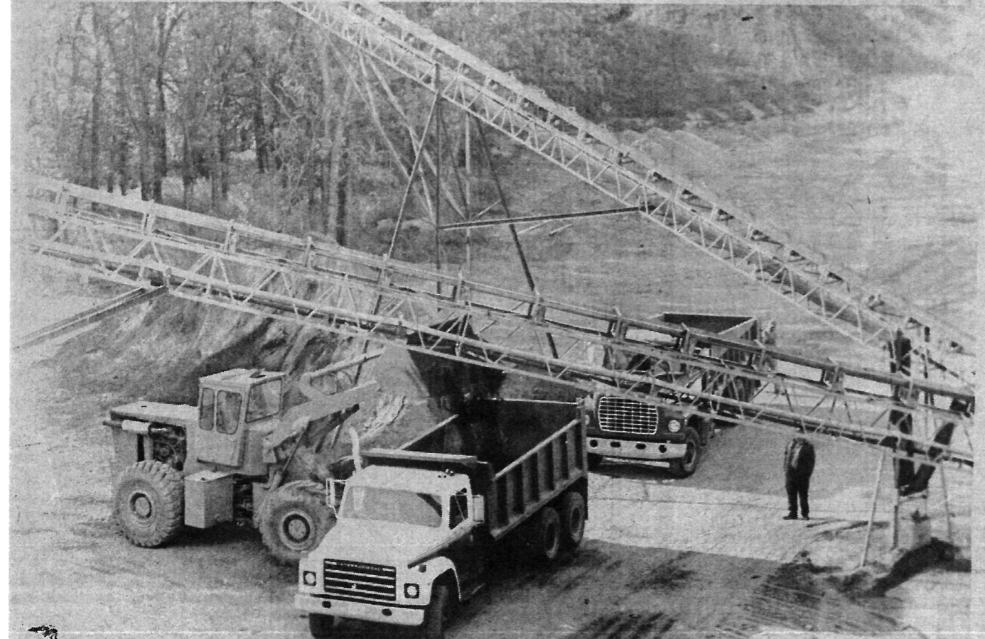
LOADING —Crews were busy last week loading up this Class 5 gravel for some road construction going on in New York Mills. These are two of the seven big dump trucks operated by Ottertail Ready Mix. (Chuck Johnson photo)
