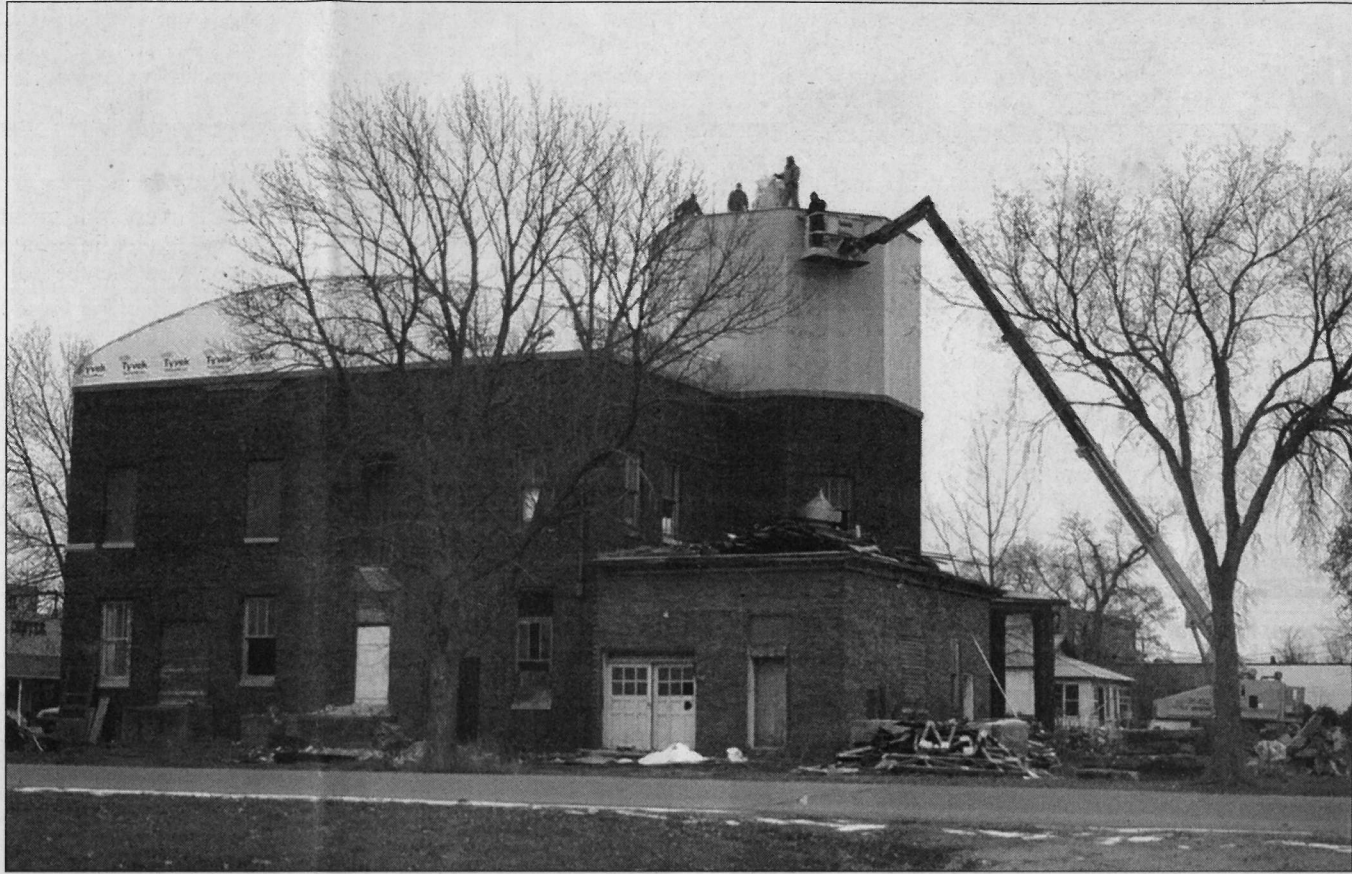
A group from Firestarters Ministries works to finish off the octagonal tower on the historic Ottertail creamery building before winter hits.
